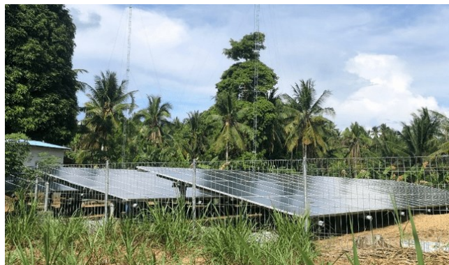
Figure 2. Solar Power System of Miang Island Village
